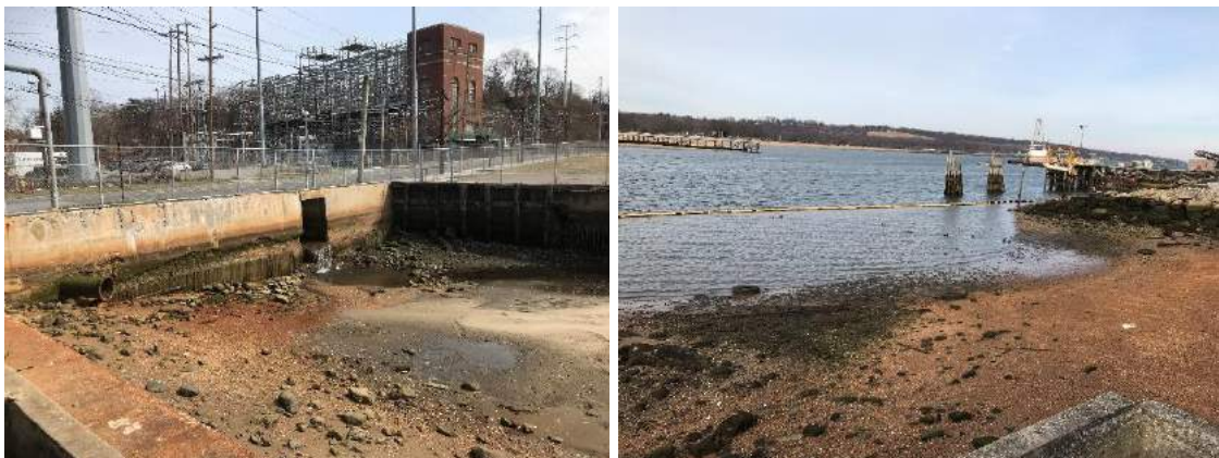
Powerhouse drain (CSHH #14A) at low tide (l) and view looking north west beyond adjacent fuel terminal dock (r) (photos by Michelle Lapinel McAllister, 3/20/20 and 5/27/20, respectively)
