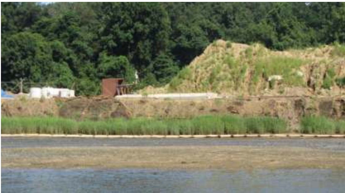
Nearly 3.5 inches of rainfall on July 22-23 caused local flooding, stormwater runoff, and a washout of newly planted wetlands along Glen Cove Creek (photo by Carol DiPaolo, 7/24/19)
