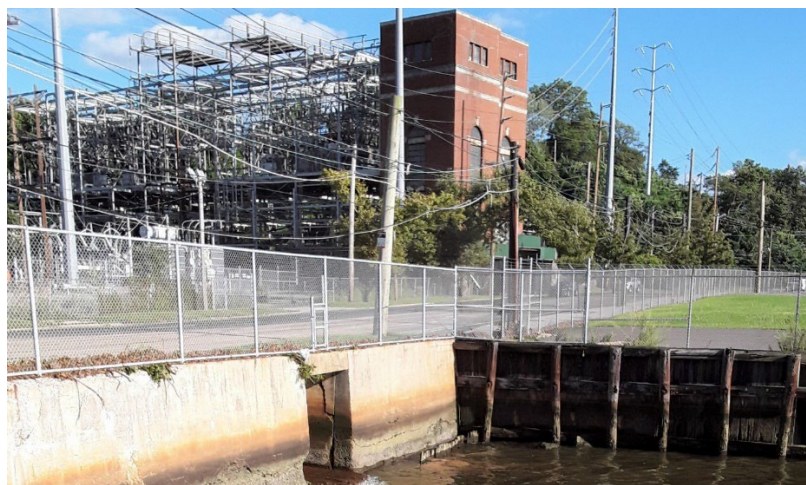
CSHH #14A, powerhouse drain outfall, adjacent to lot that was the site of the old powerhouse building (photo by Carol DiPaolo, 9/2/21)
