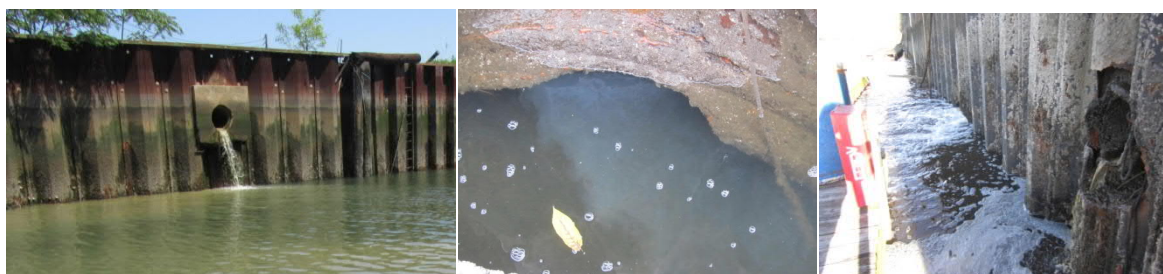
Brown discharge from north bulkhead outfall, Glen Cove Creek (l); white discharge from CSHH #10 (center); brown discharge at CSHH #9 (r) (photos by Carol DiPaolo, 5/17/17 and 10/11/17, respectively)
