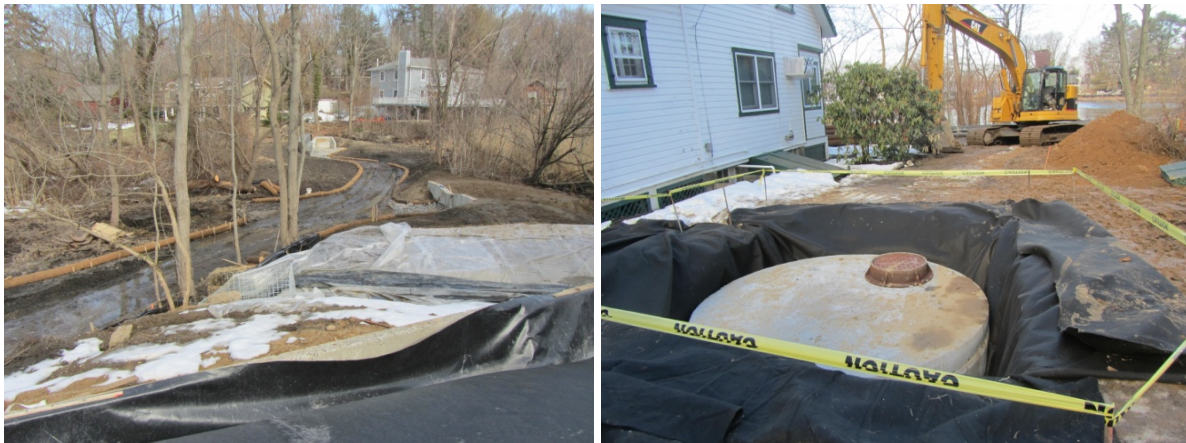
Scudder's Pond restoration and construction work: coir banks for stream from upper pond (l) and new stormwater basin for country club cottages (r) (photos by Carol DiPaolo, 3/11/14)
