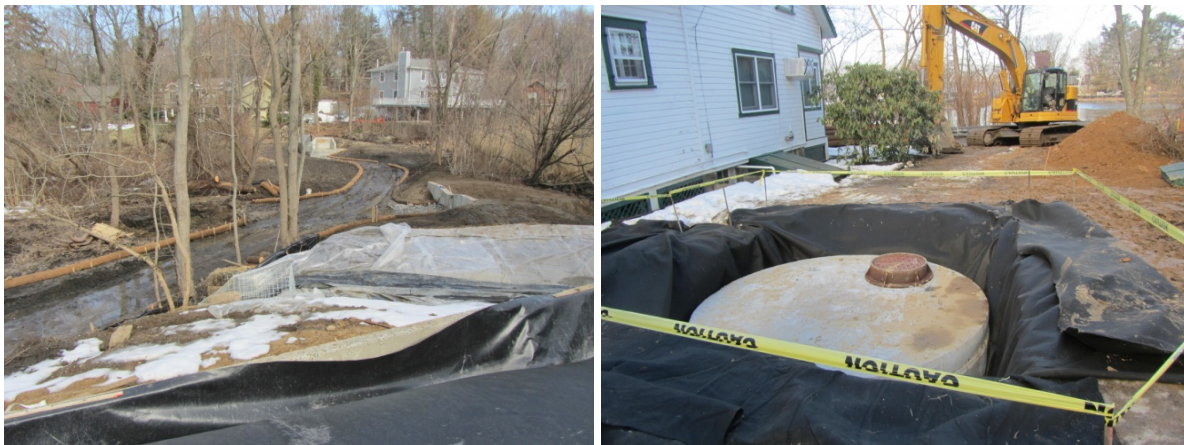
Scudder's Pond restoration and construction work: coir banks for stream from upper pond (l) and new septic tanks for country club cottages (r) (photos by Carol DiPaolo, 3/11/14)
