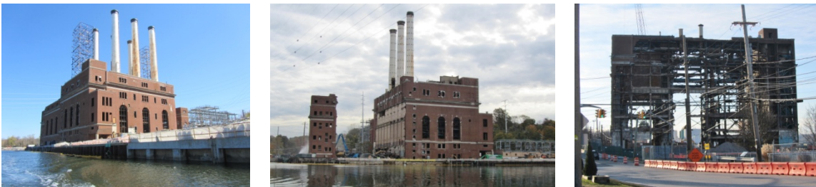
Demolition stages of the Glenwood Landing power plant from April to December 2014 (photos by Carol DiPaolo)
