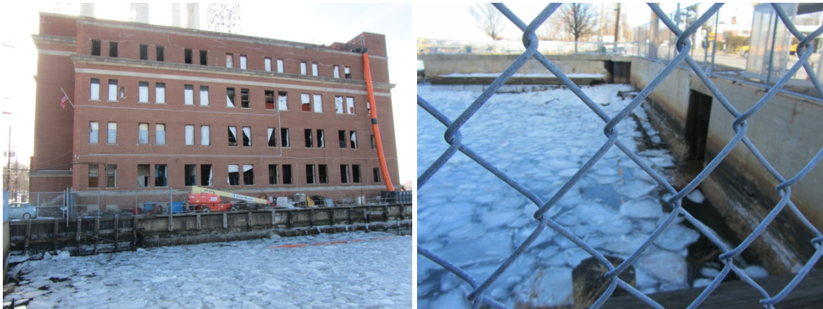
Power plant substation demolition (l) and snowy, cold weather made sample collection difficult at CSHH #14A (r) (photos by Carol DiPaolo, 1/28/14)
