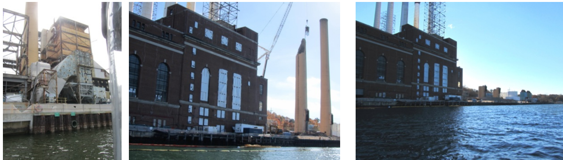
Demolition stages of the Glenwood Landing power plant from May to November 2013 (photos by Carol DiPaolo)
