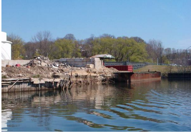
Collapsed bulkhead on north side of Glen Cove Creek (4/18/08) (photo by Carol DiPaolo)
