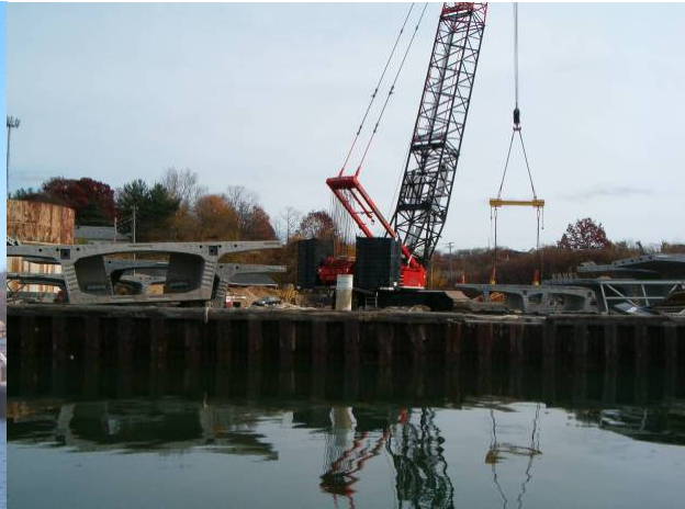
Girders used for the Roslyn viaduct at the staging area along the harbor (11/12/08)(photo by Carol DiPaolo)
